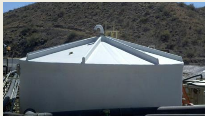
Spend acid storage tank
