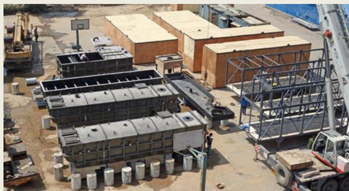
Solvent Extraction plant
