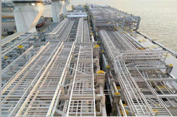
Stainless steel cable trays
