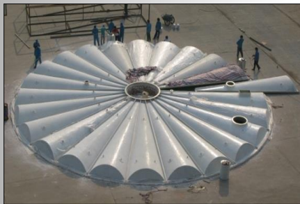
18.4 mt. dia. clarifier cover
